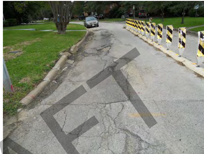
Localized Pavement Failure
