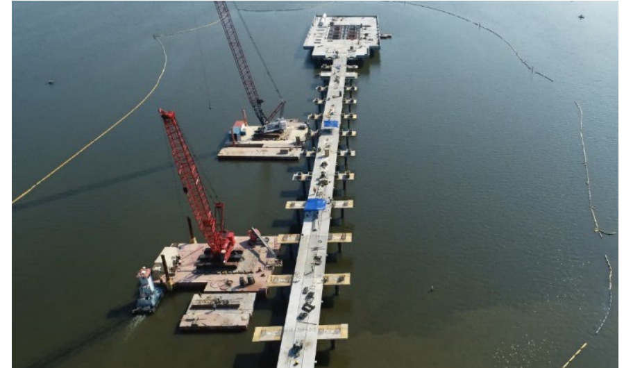
Intake Pump Station
