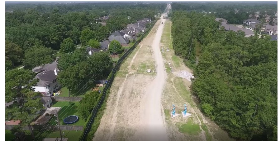
Raw Water Pipelines
