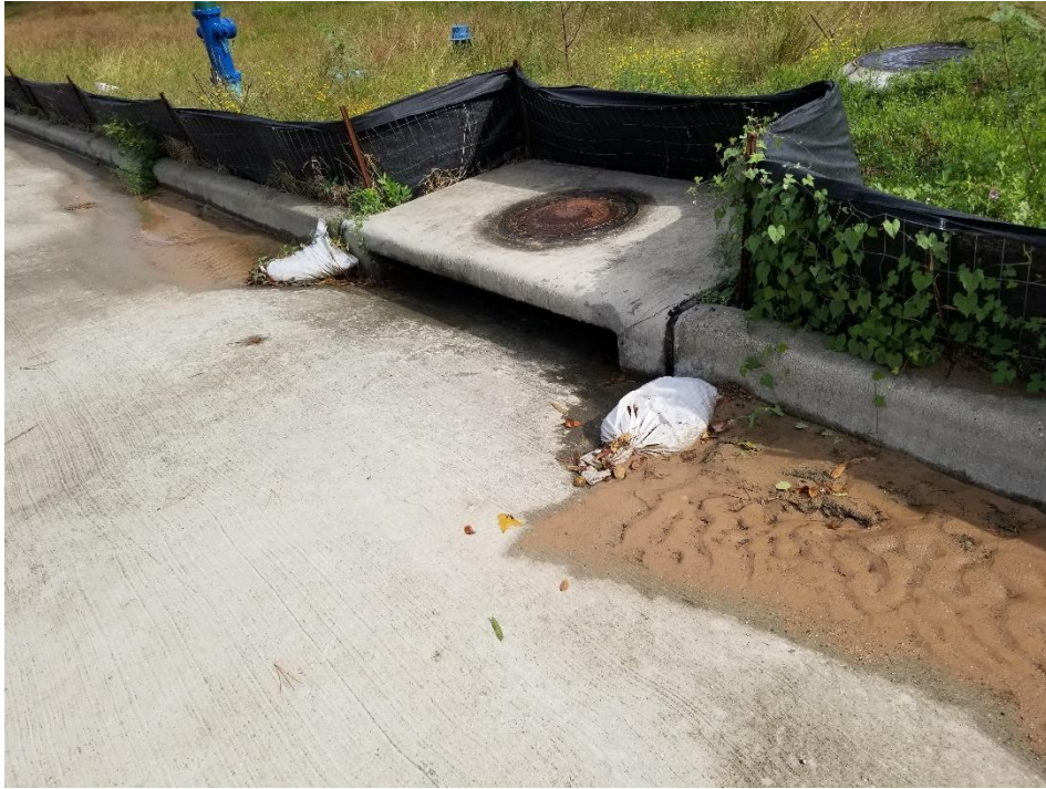
Storm Sewer Inlet on Woodland Hills Drive Note: BMP's require maintenance
