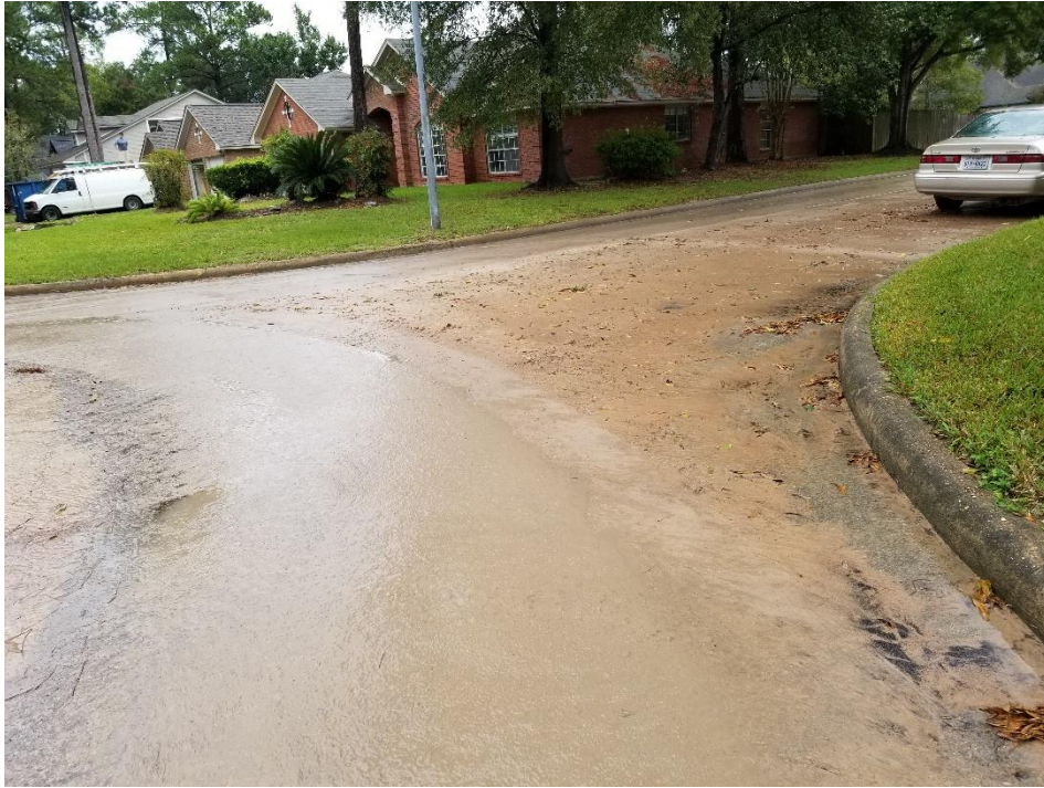
View of Sediment at Intersection of Village Springs Drive and Creek Manor Drive Note: Additional sweeping is required
