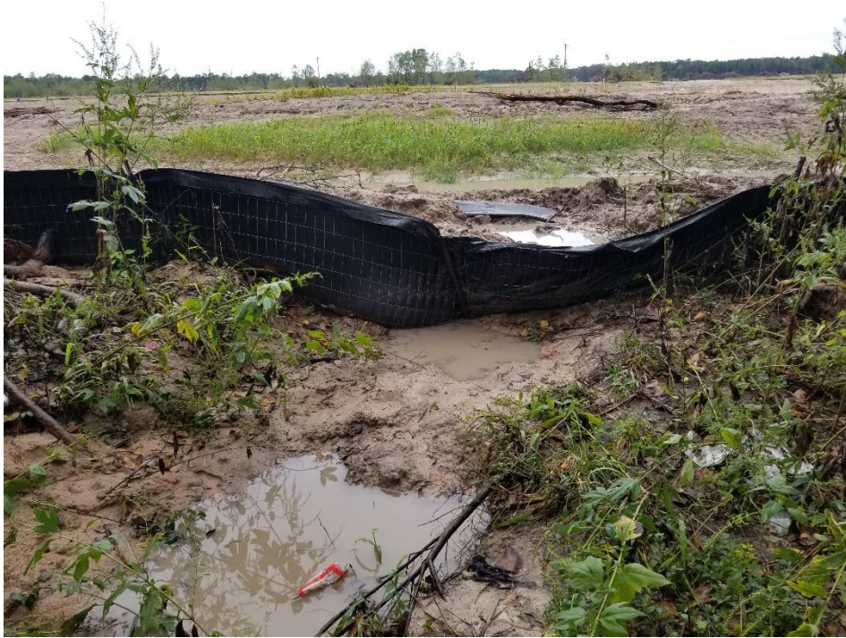
Silt Fencing Requires Maintenance
