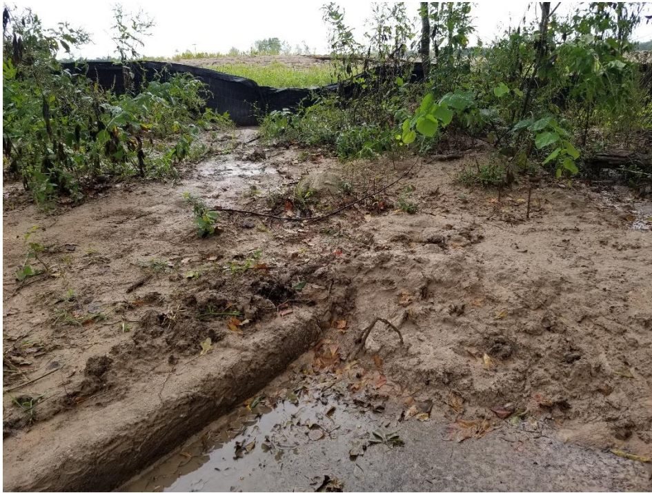
Sand / Silt on Village Springs Drive
