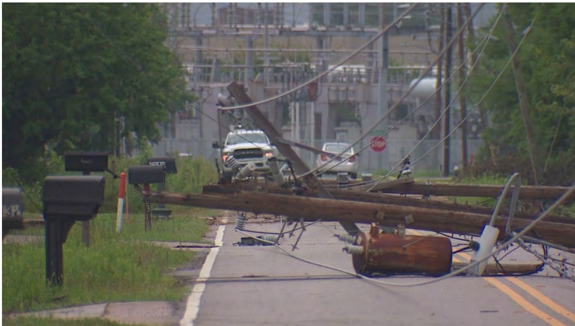
Figure 5: Infrastructure Damage – Downed Powerlines
