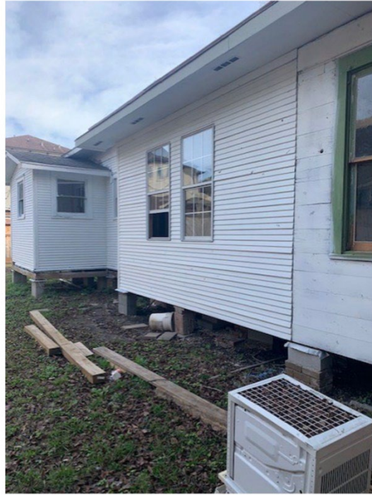
Side- west – existing. Non-original windows to be removed and replaced with windows reclaimed from rear of house; area of missing siding to be replaced with matching 117 siding
