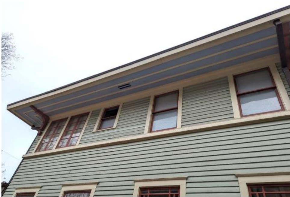
South (side) elevation, January 2024. Two center upstairs windows (one small 1/1, one larger 1/1) will be preserved and relocated to the east (front) and west (rear) walls of the bathroom addition.
