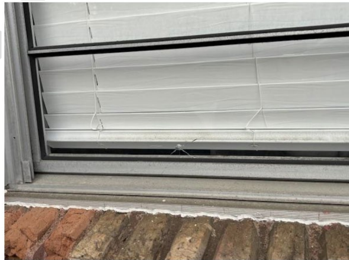
A2 – Window sustained damage as a BB pellet went straight through glass
