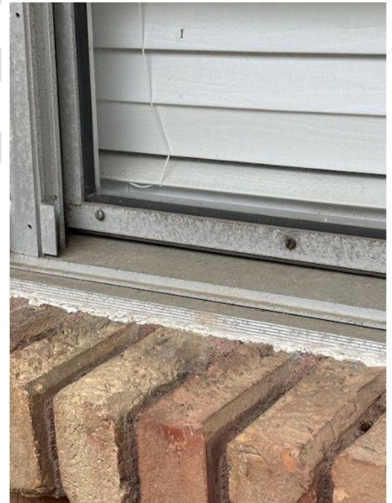
A3 – Window does not seal and cannot close properly on all sides, leaving a gap which allows debris and increased noise
