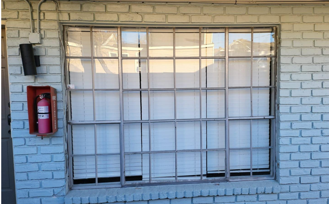
Window Example Before Replacement
