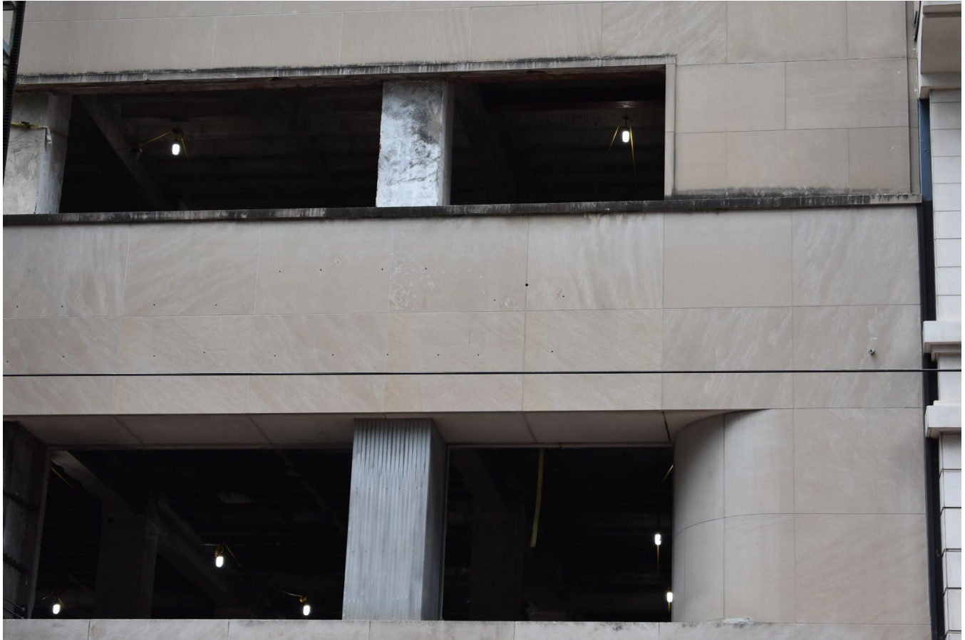
Photo 5: East (front) elevation facing Main Street. Detail view of second and third floor transition. Camera facing northwest. Photo by applicant, 2024.
