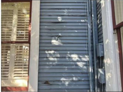
Large amount of wood rot observed around exterior of house
