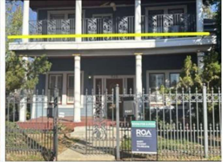
Balcony has significant sagging recommend further investigation/repair as needed
