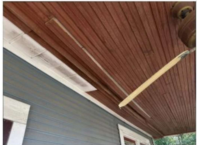
Loose ceiling material observed on the balcony
