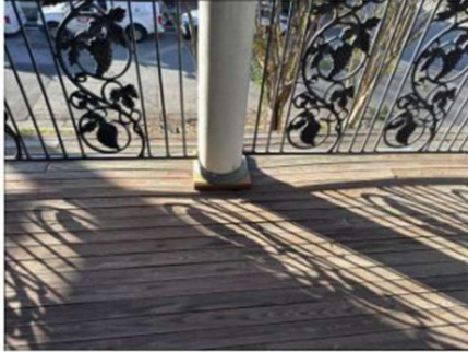
Balcony decking material is dilapidated
