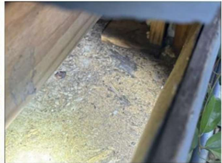
Evidence of Drywood termite activity below glass block window/stair landing
