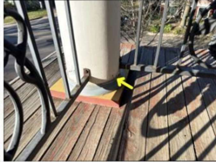
Base of column/post is deteriorated
