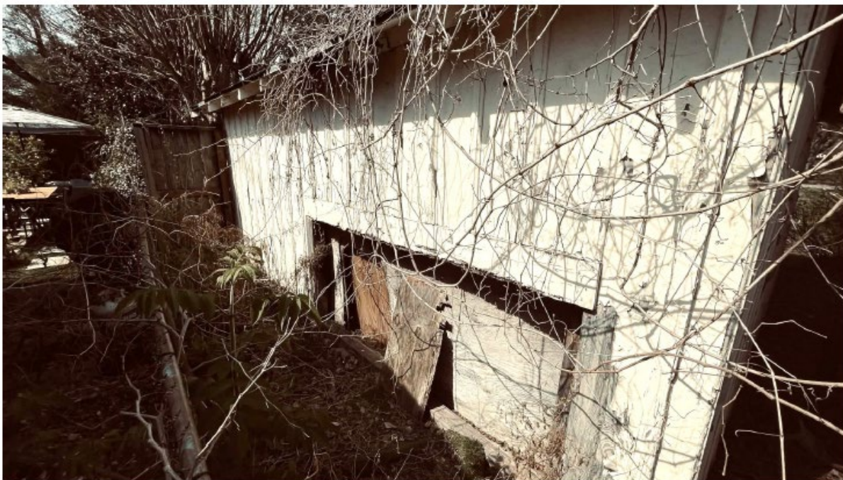
South elevation of garage. A previous owner had built a metal box extension through the back wall of the garage to get a large car in. It has disintegrated.
