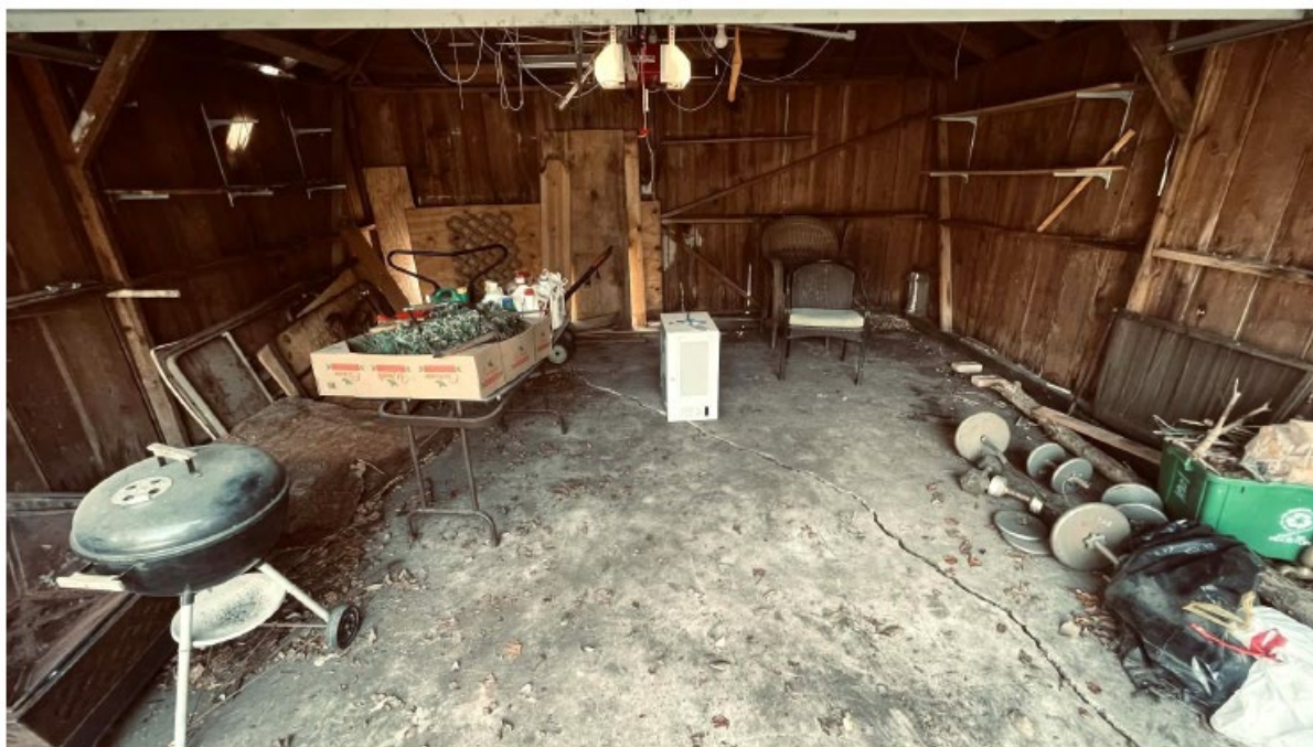
Interior of garage. Previous owner had unreinforced concrete floor poured and garage now holds water after moderate rain.
