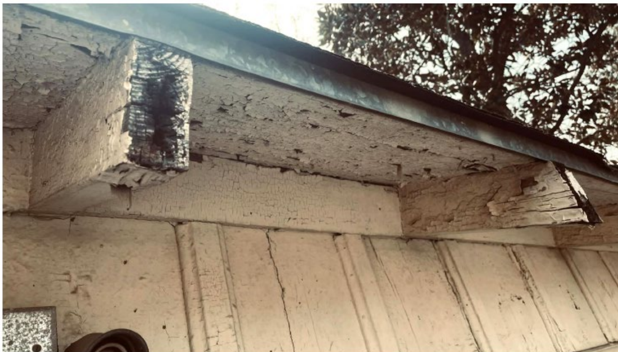
North open eave joists rotting.
