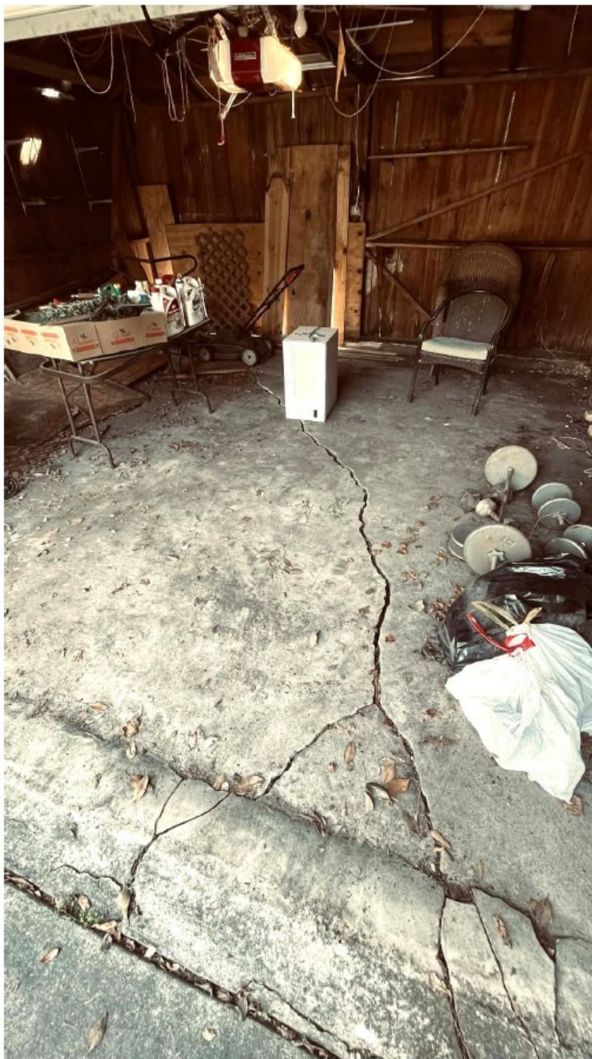
Large cracks in unreinforced concrete in garage interior.
