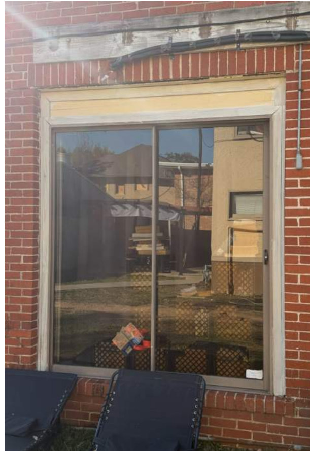
SIDE (EAST ELEVATION) #11 TO BE REMOVED, NOT ORIGINAL
