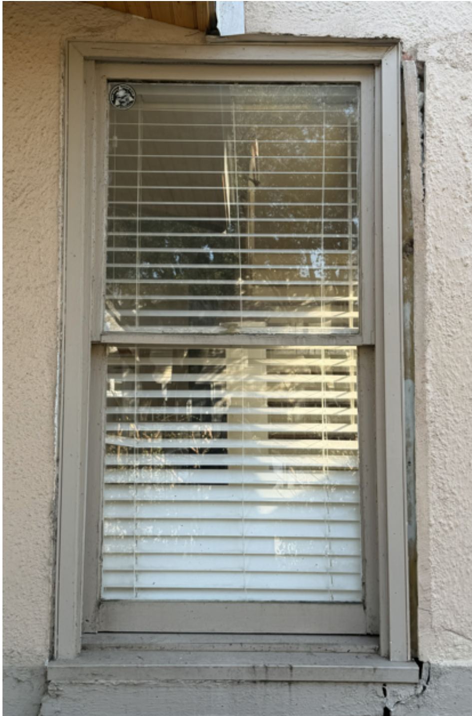
EXISTING 503 SUL ROSS SINGLE HUNG WOOD WINDOW WITH SURROUNDING WOOD TRIM AND WINDOW STOOL
