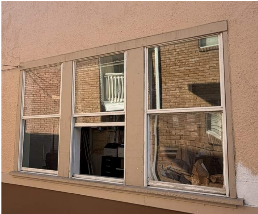
SIDE (EAST ELEVATION) #13, #14, AND #15 TO BE REPLACED WITH NEW TO MATCH EXISTING, ALL 3 NOT ORIGINAL
