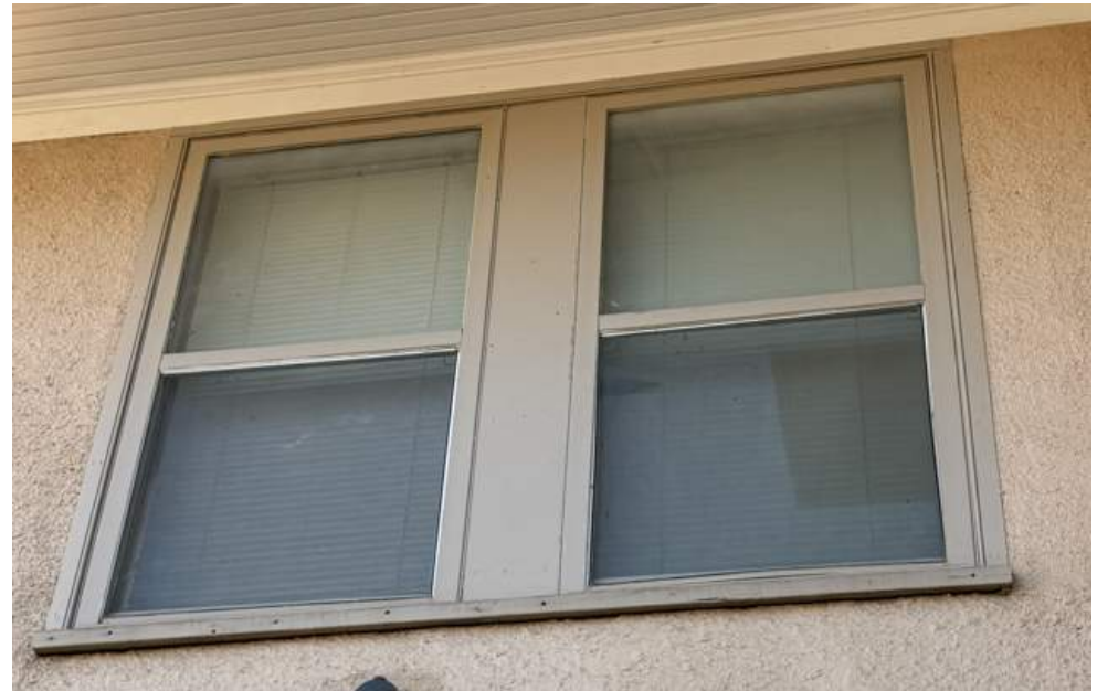
FRONT (NORTH ELEVATION) #7 AND #8 TO BE REPLACED WITH NEW TO MATCH EXISTING
