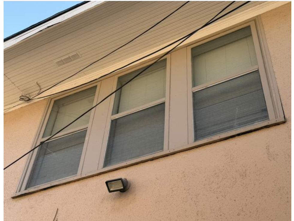
SIDE (EAST ELEVATION) #16, #17, AND #18 TO BE REPLACED WITH NEW TO MATCH EXISTING, ALL 3 NOT ORIGINAL
