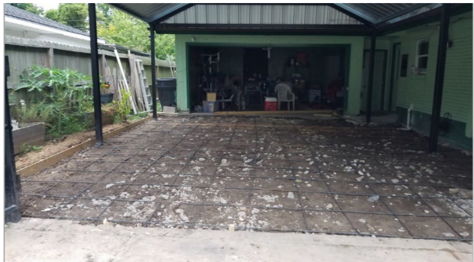
Figure 4 - Violation Notice July 2020
